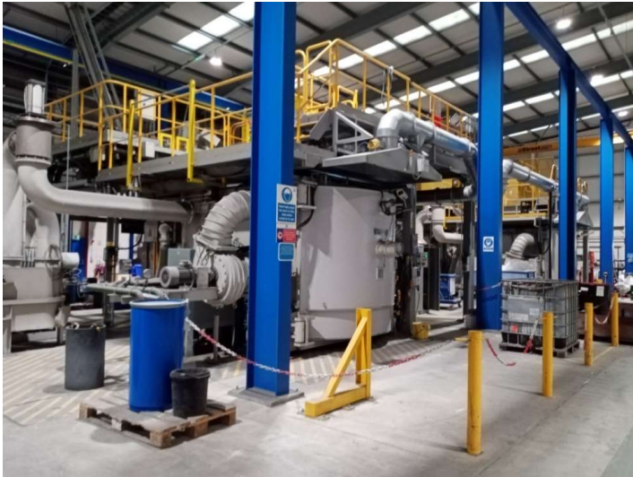
Strip cast equipment installed in LCM
